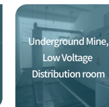
Electrical Equipment Room Decompression Room
